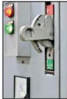
Main disconnect switch
